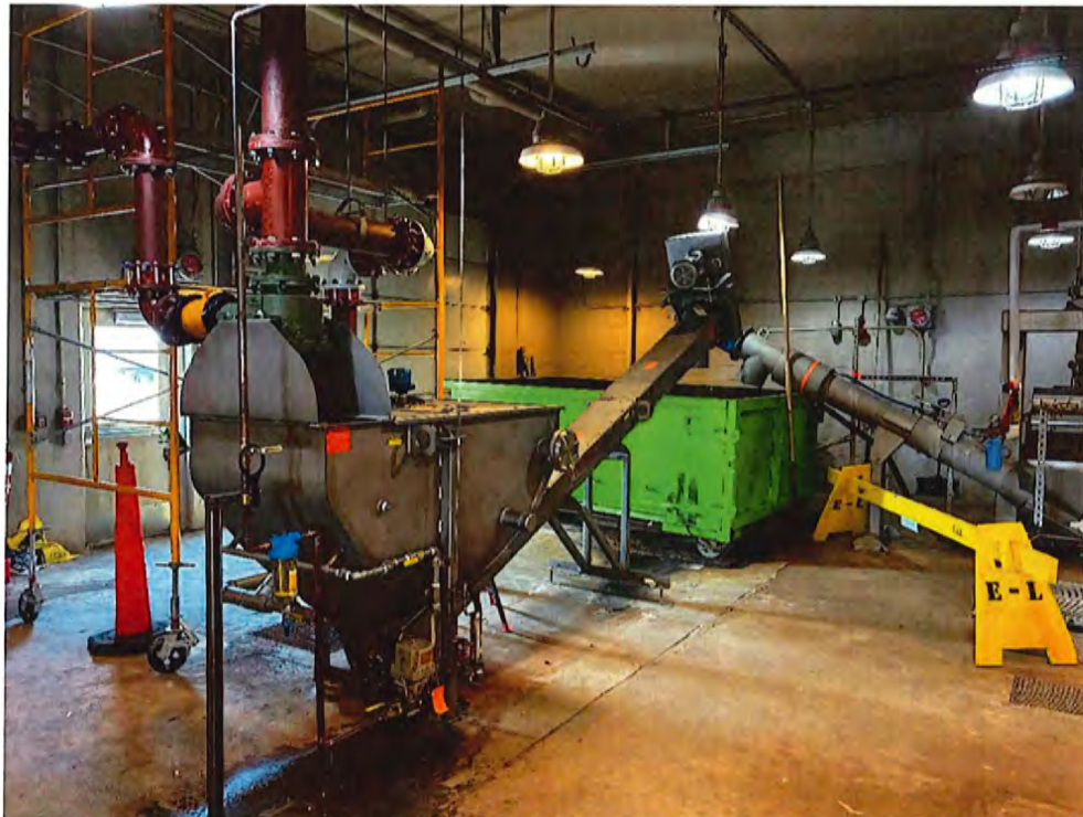
Figure 2 - New Grit Removal Equipment Installed.
